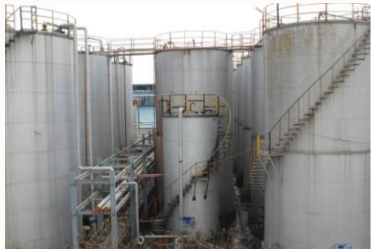
Fig.6.3 Dedicated Storage Tanks
