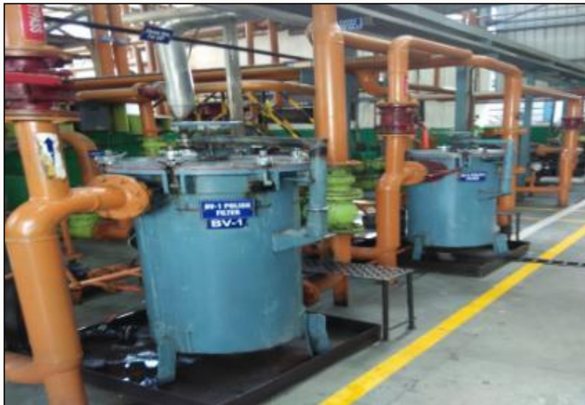
Fig.2.21. Rust free/ non corrosive coating of equipment's
