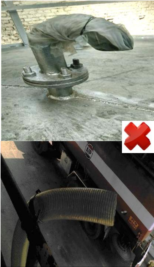
Fig.6.4 Open hose pipe (chances of cross contamination)
