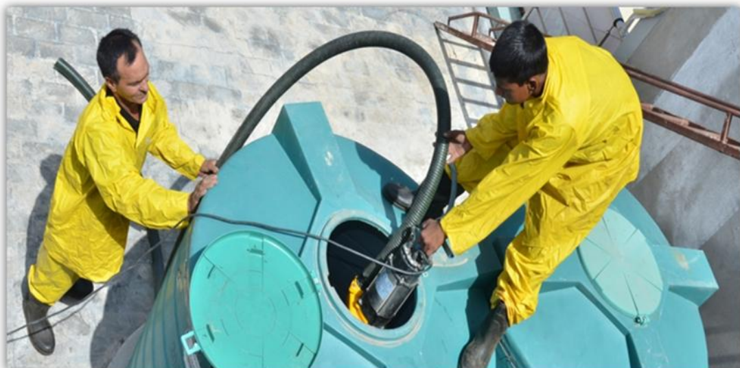
Fig.2.25 Routine cleaning of water storage tanks
