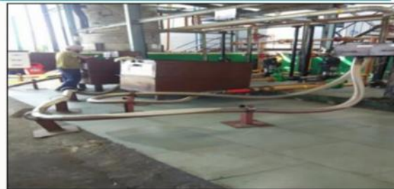
Fig.3.2 Hanging of flexible pipes for ease of cleaning
