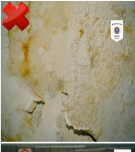
Fig.2.9 Fungal growth on the walls
