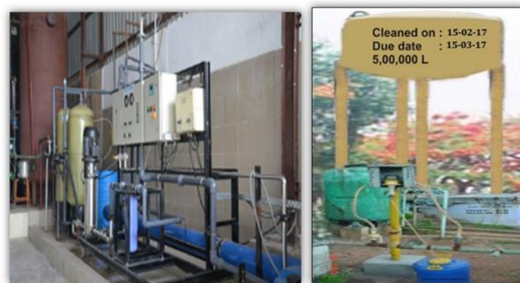
Fig.2.26 If required waste water disposal system/effluent treatment plants shall be put in place.
