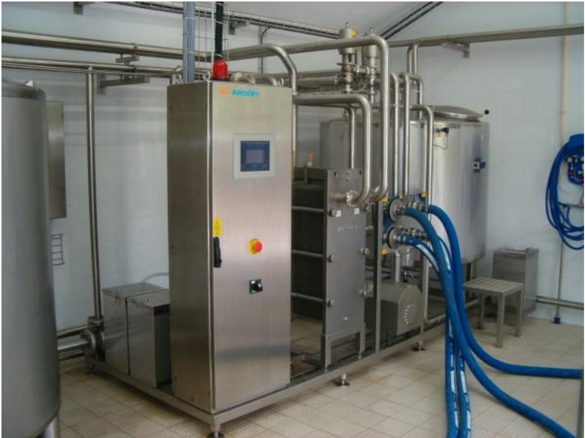
Fig.3.3 Illustrative of fixtures and equipment's in the manufacturing plant
