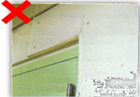
Fig.2.8 Cracks allow bacteria and moulds to accumulate.
