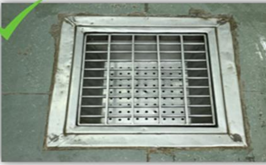
Fig.2.17 Drains should be covered to prevent insects and rodents
